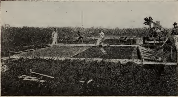
Fig. 3.—Poultry house floor and foundation under construction. Note the form construction and that the floor and foundation are being poured together.
